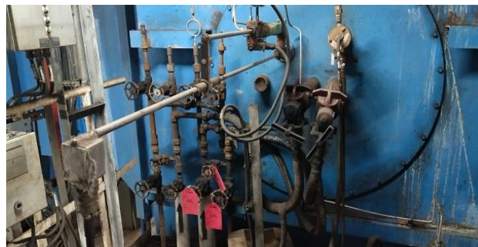
Gambar 2. Area Burner Auxiliary Boiler (Sumber: Dokumentasi Pribadi)
