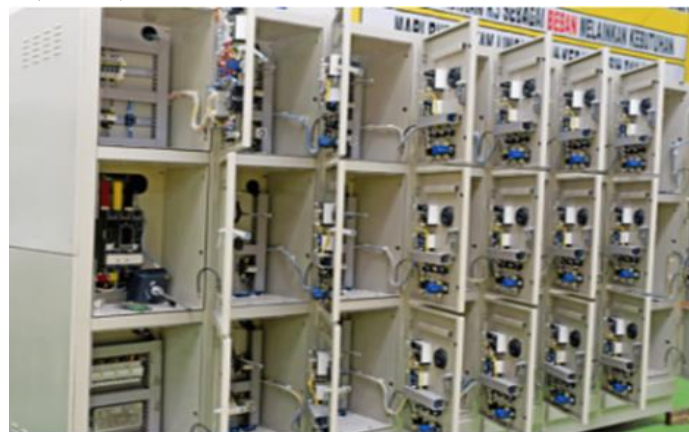
Gambar 1. Panel MCC (Sumber: Indonetnetwork)
